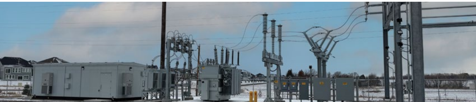
The new South Dayton substation was energized in February 2024.
