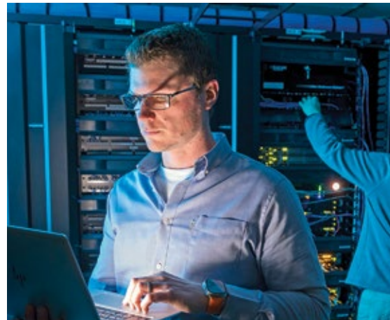
Cyber Security Architect Bryan Dumire in the campus data center.
